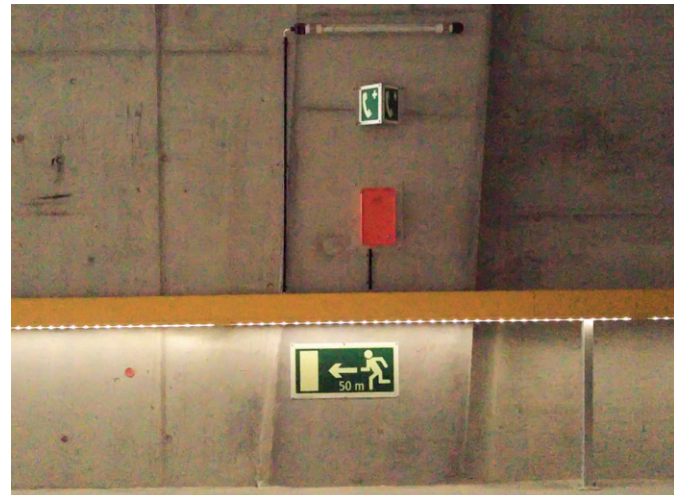
Direction display for emergency escape route
